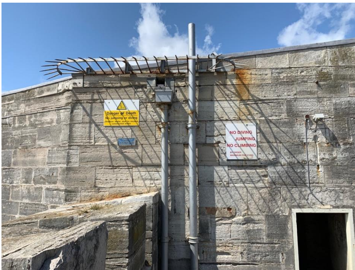
Photograph 3 Restrictive Bars and Safety Signage, Flanking Battery
